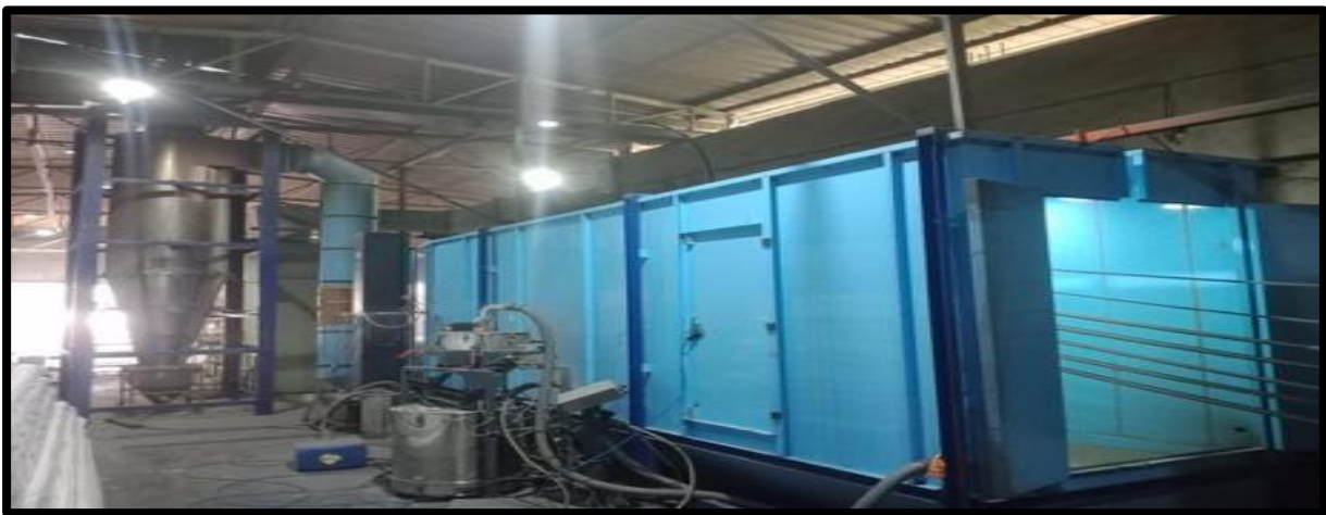
AUTOMATIC POWDER COATING SYSTEM
