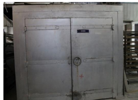
Gas oven – the bricks are dried in our gas oven before going for firing to remove the moisture
