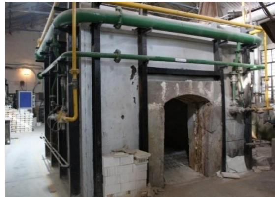
Kiln –D (7 ton)- natural gas fired downdraft firing the material
