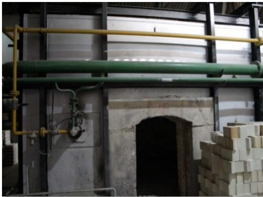
Kiln –B (10ton)- natural gas fired downdraft kiln for firing the material
