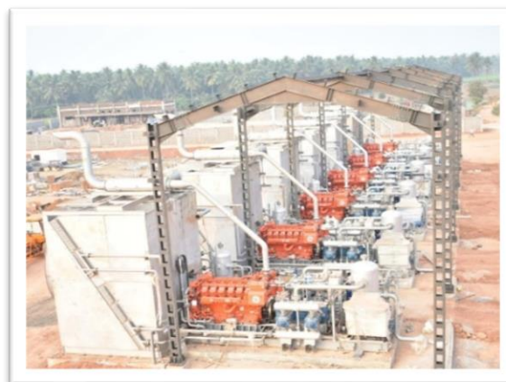
Gas Compression Station, GITL Tadepalligudem
