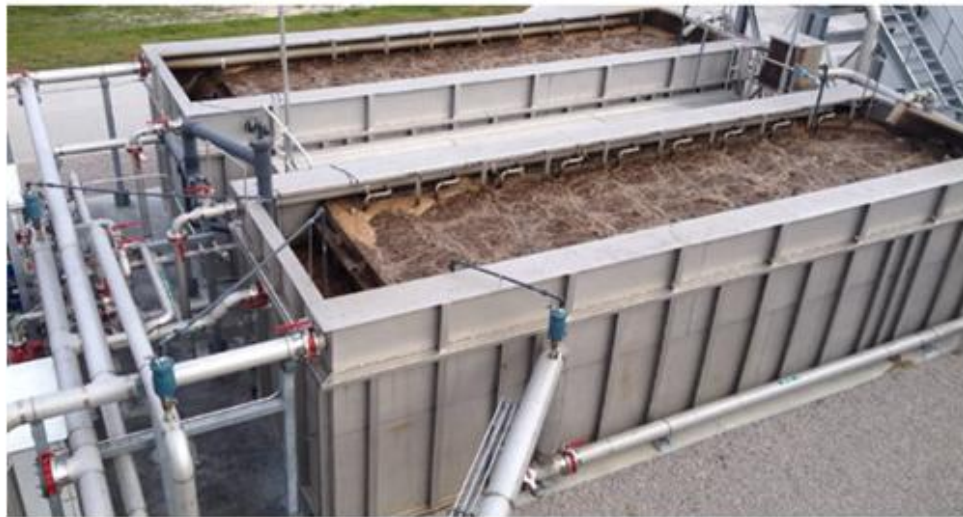
Note(s): Image represents secondary treatment which includes biological degradation of organics matter
